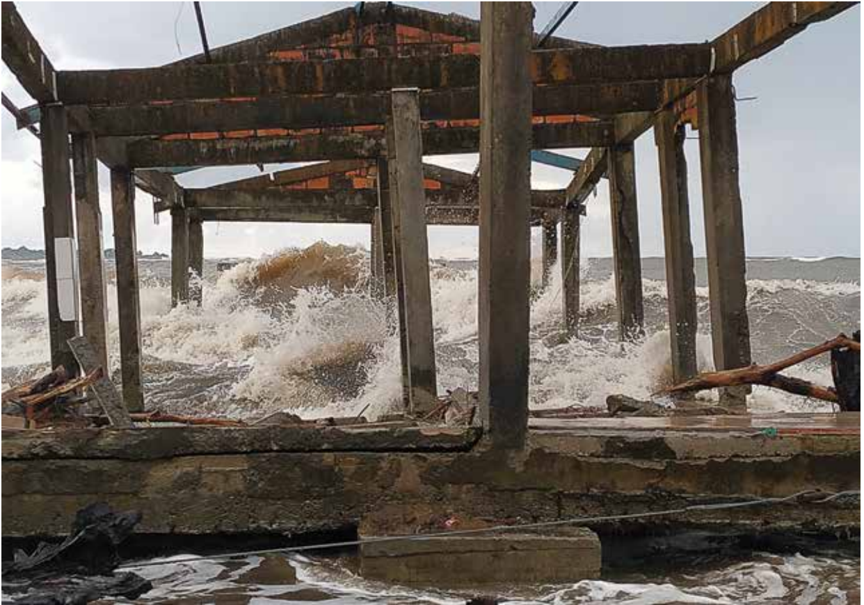
Photo: Infrastructure damage on the Punta Soldado Island, 2019
